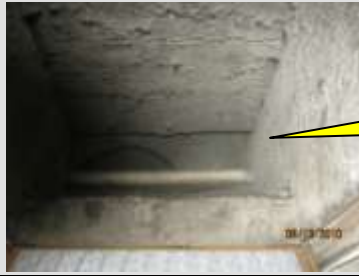
Dust buildup inside return air
